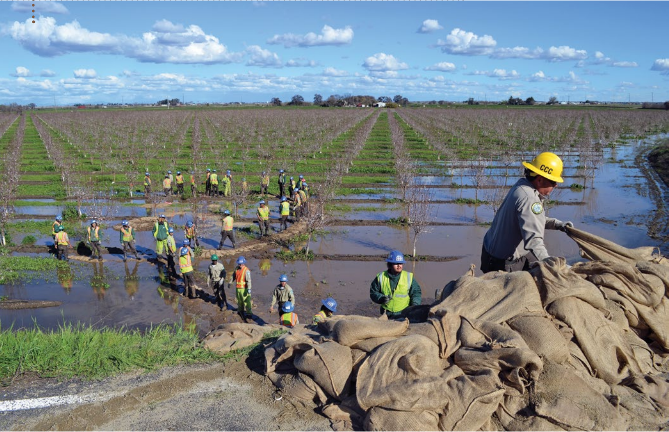
U.S. Army Corps of Engineers Sacramento District make repairs to the San Joaquin River Levee in California in February 2017.
